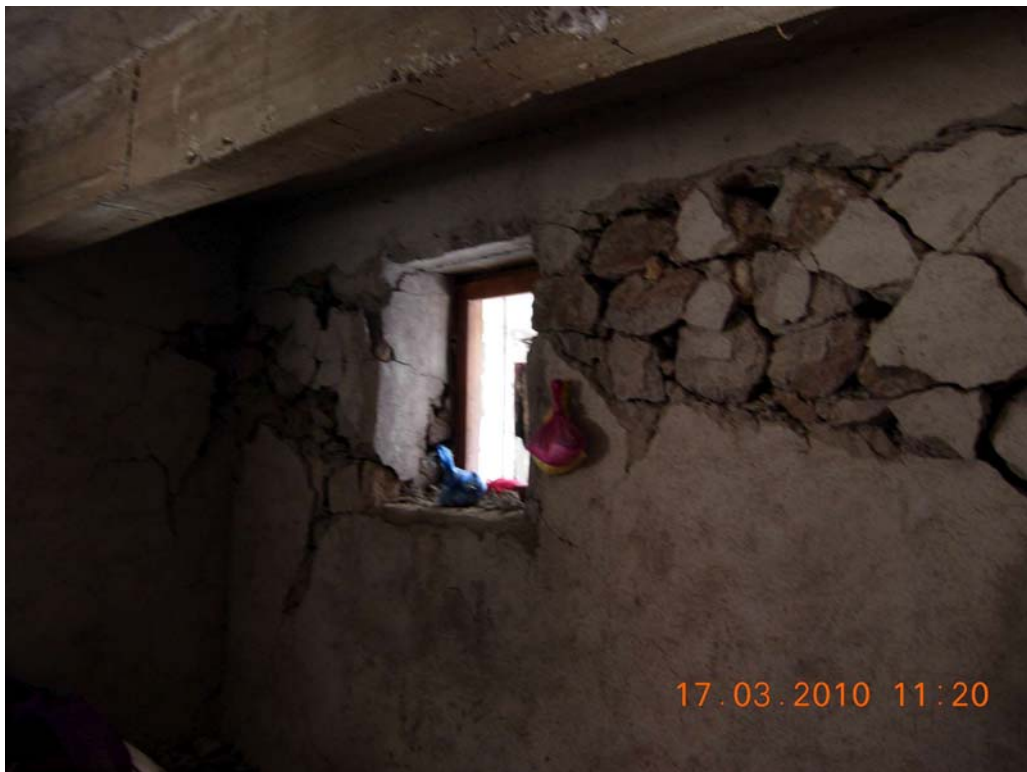
Figure 46: Inside view of two storeys mixed structural system, RC beam, RC slab, heavy stone wall, Okular village
