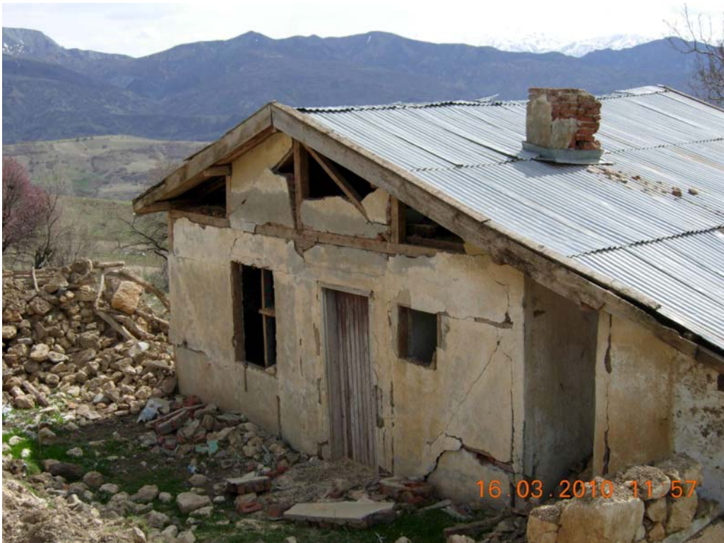
Figure 60: Refractory brick houses built after 1971 Bingol earthquake, Yukarıkanatlı village
