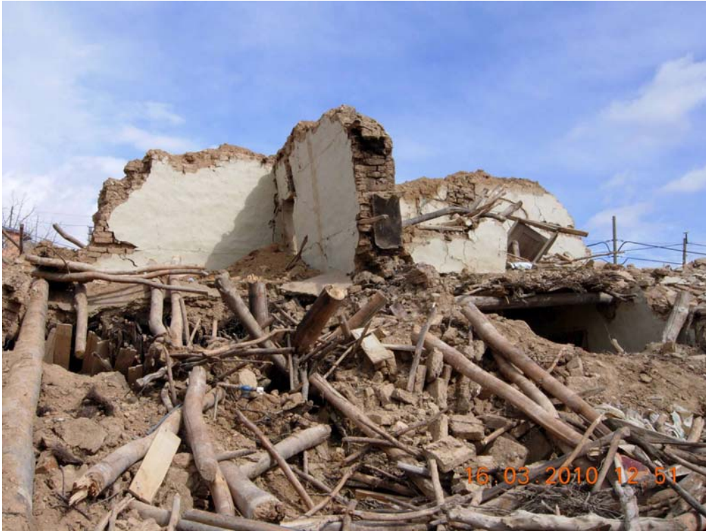
Figure 23: Two storey soil brick house with a stall in the ground floor, front view, Okular
