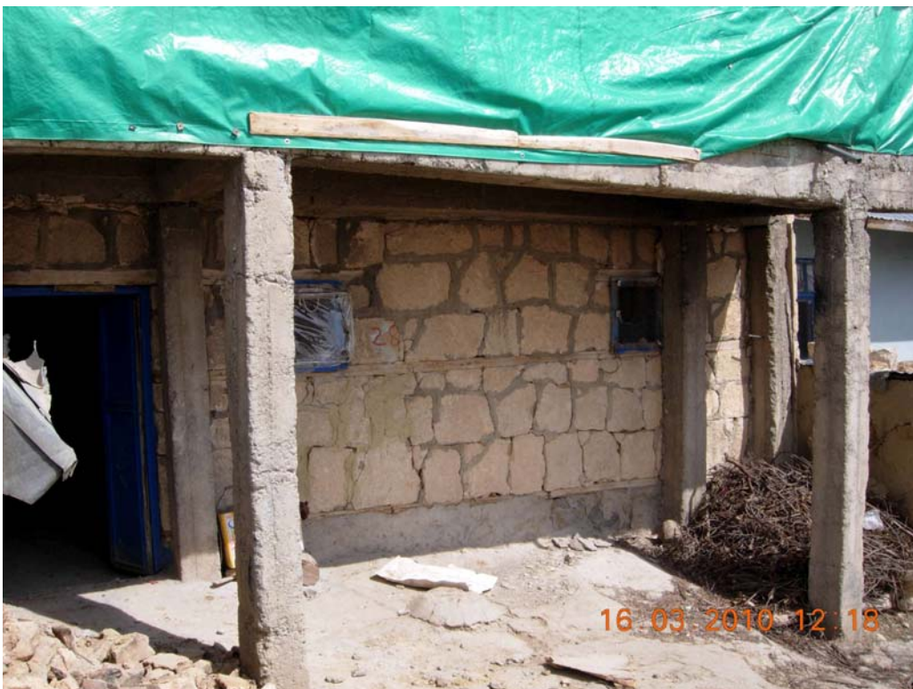
Figure 29: Ground floor of two storey light stone house, with a stall as ground floor, Okcular village
