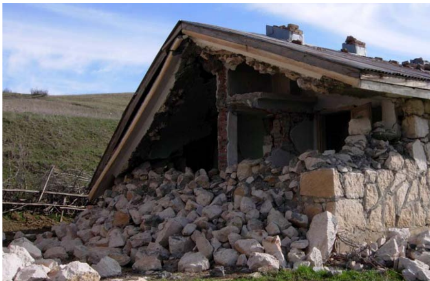
Figure 75: Out of plane failure due to lack of integrity between soil brick and stone walls in one story house, Aşağıkanatlı village
