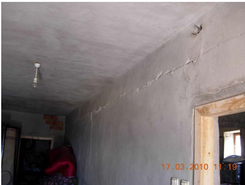
Figure 40: Inside view of two storeys mixed structural system, RC beam, RC slab, infill brick wall, Okcular village
