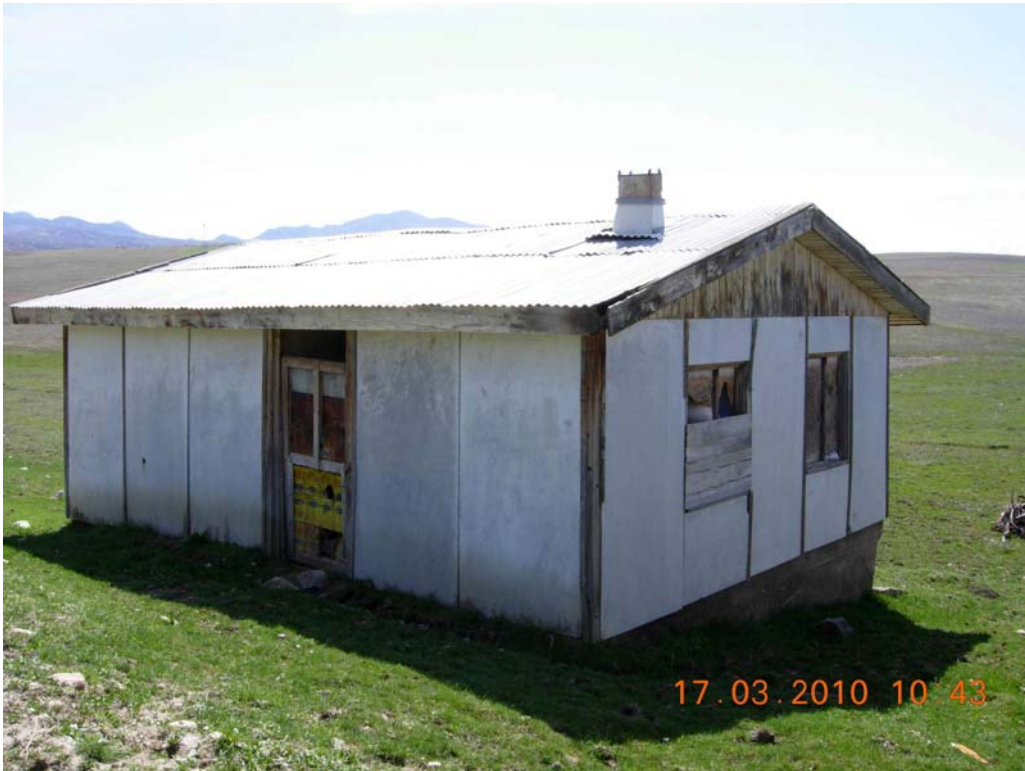
Figure 62: Prefabricated panel houses built after 1971 Bingol earthquake, being used as storage room, Incedal village
