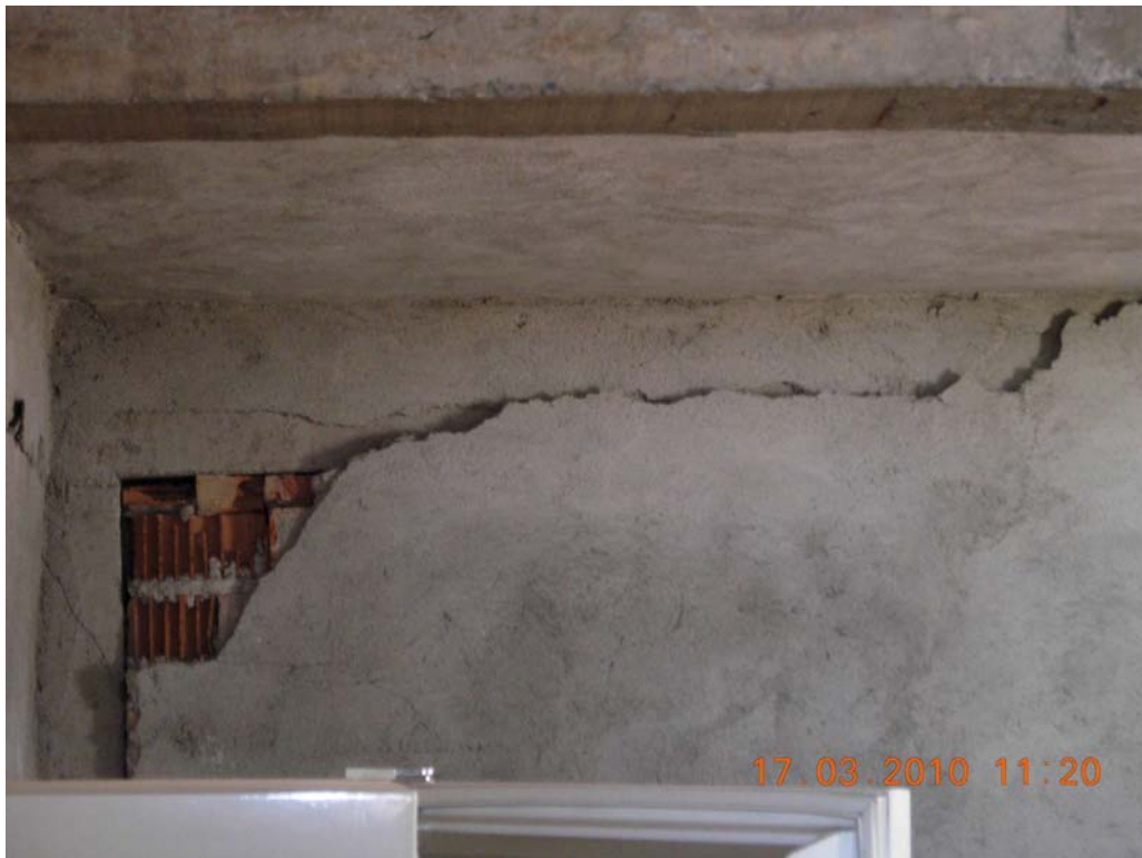
Figure 44: Inside view of two storeys mixed structural system, RC beam, RC slab, heavy stone wall, Okcular village
