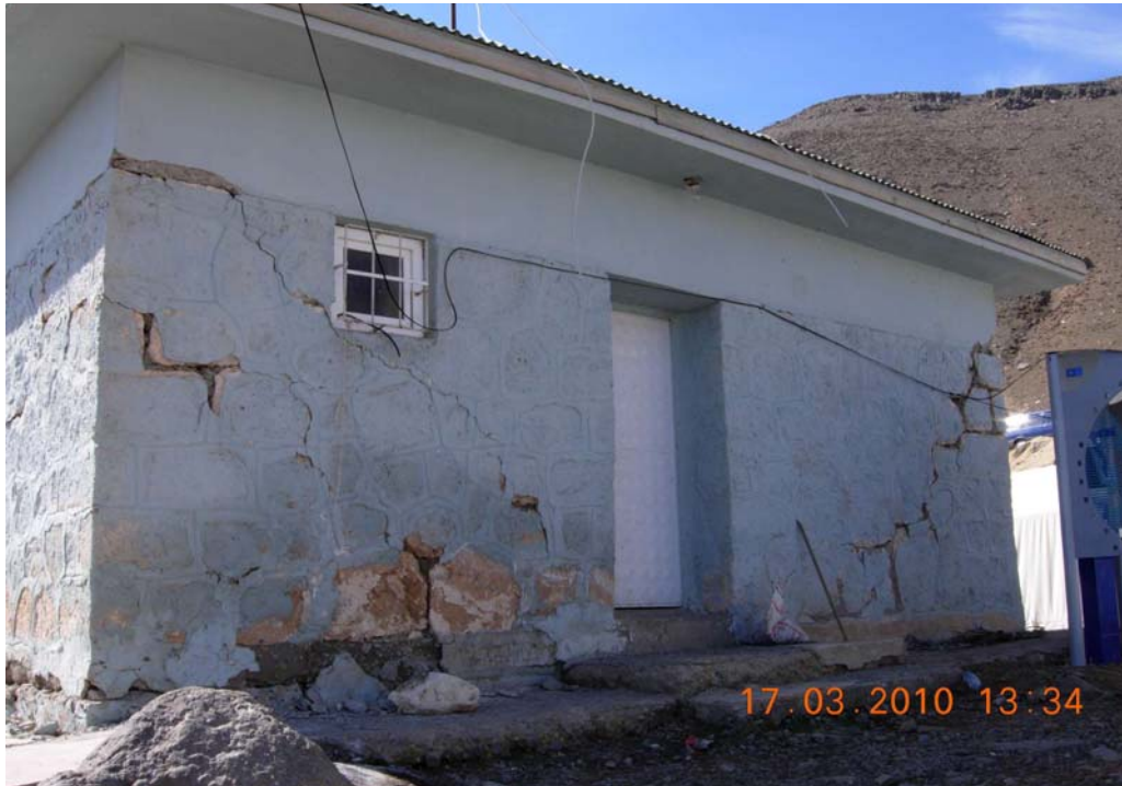
Figure 80: Wide cracks following the mortar, Yukarıdemirci village
