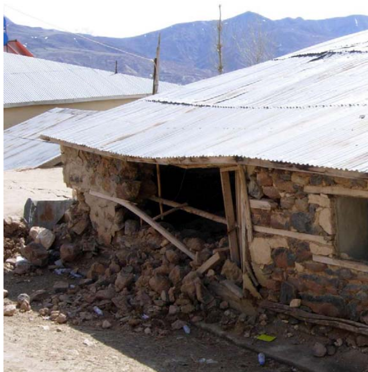
Figure 79: Insufficient interlock among the rounded stones, Okçular village
