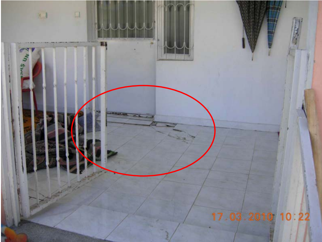
Figure 69: RC house, built by government, after 2003 Bingol earthquake, Incedal village
