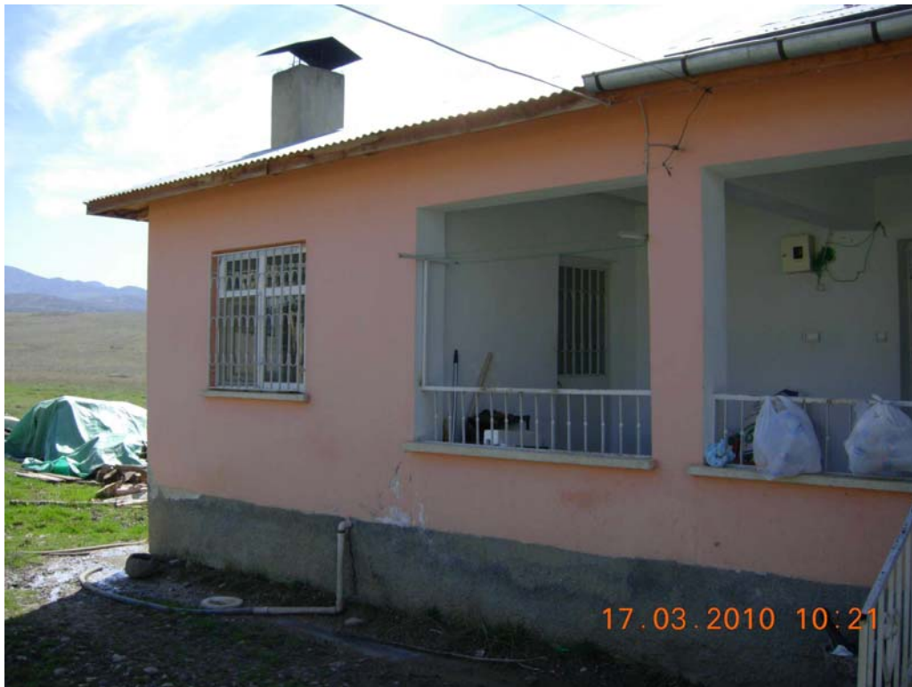
Figure 68: RC house, built by government, after 2003 Bingol earthquake, Incedal village
