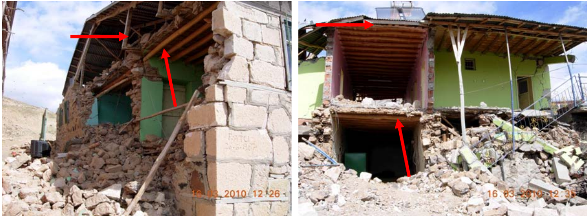
Figure 76: Out of plane failure in two story stone houses, Okcular village, in both pictures “lack” of rigid diaphragm effect is visible, as well as bad integrity of walls constructed with different materials.
