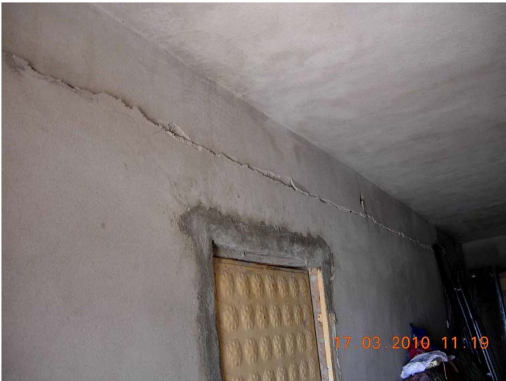
Figure 42: Inside view of two storeys mixed structural system, RC beam, RC slab, heavy stone wall, Okular village
