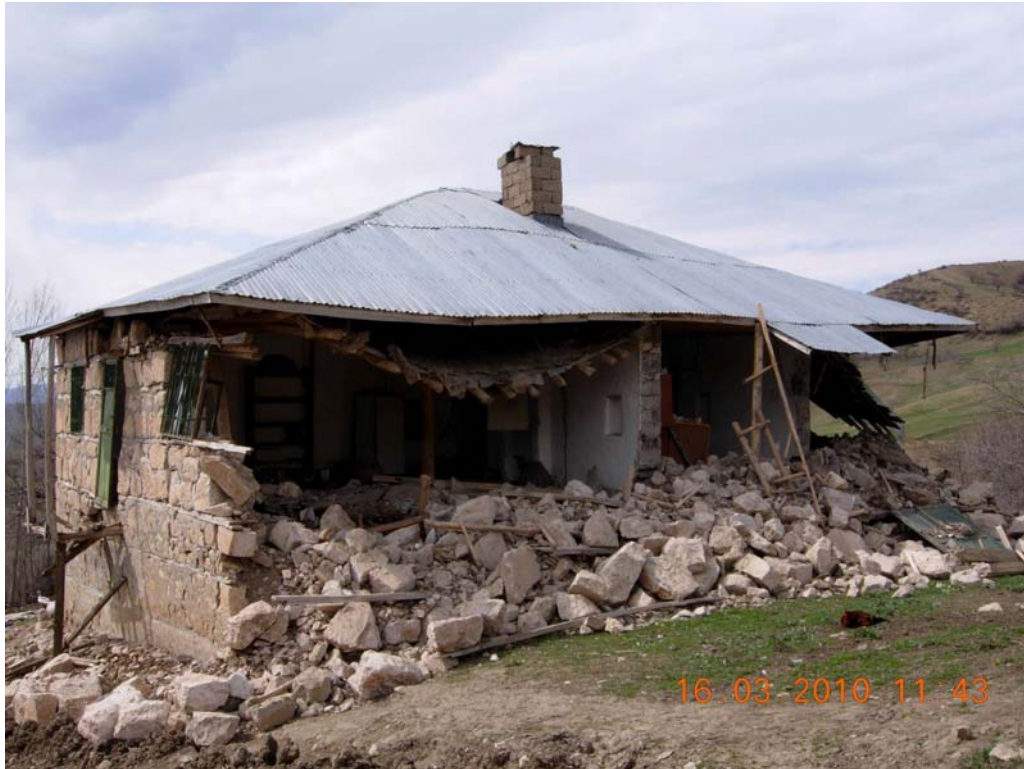
Figure 77: Out of plane failure in one story stone house, Yukarıkanath village
