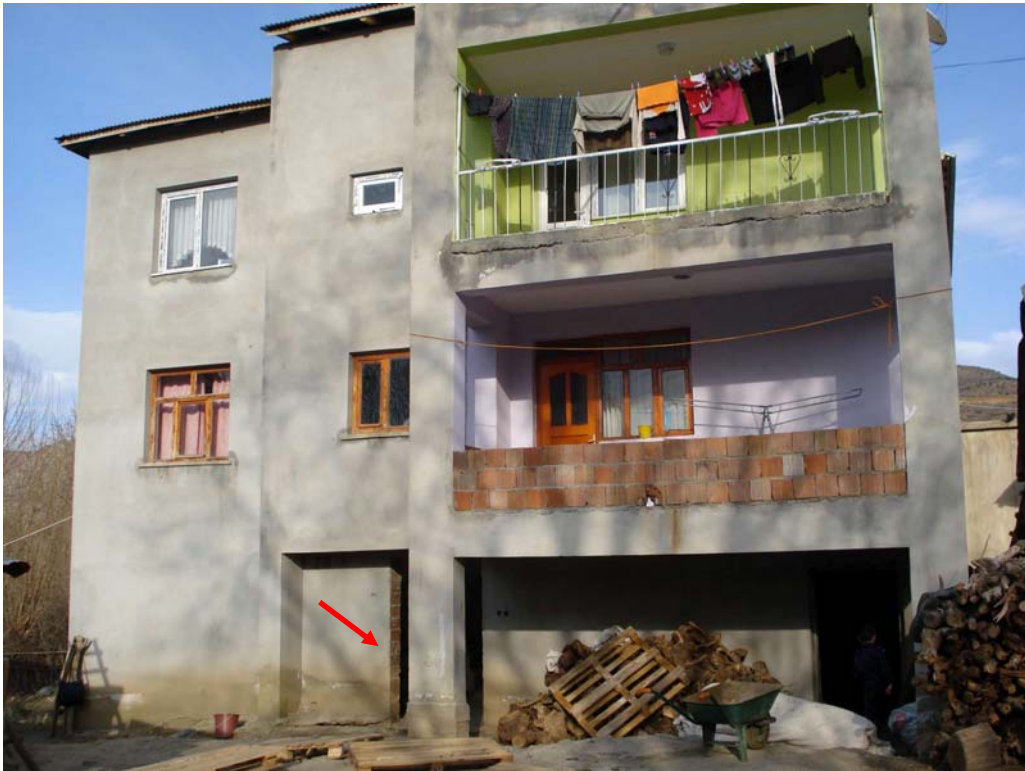
Figure 48: Outside view of three storey house, infill bricks filled with concrete as load bearing walls, in Okular
