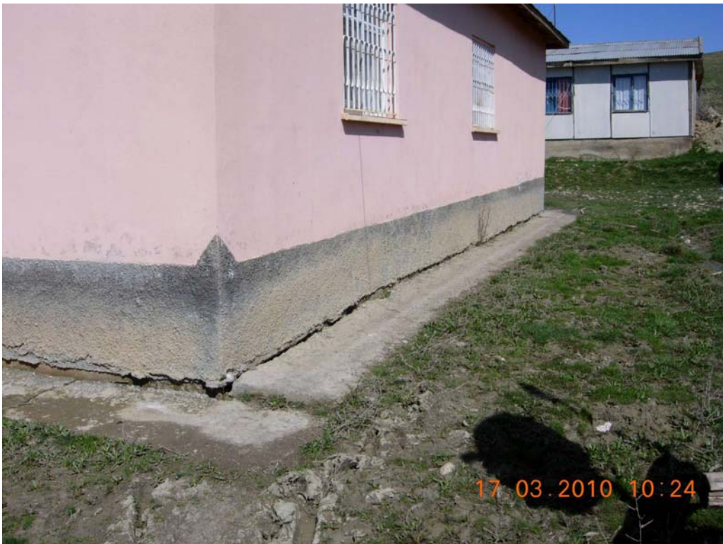
Figure 70: RC house, built by government, after 2003 Bingol earthquake, Incedal village
