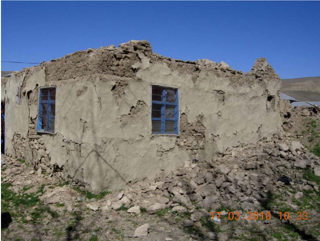
Figure 19: One storey soil brick house in Incedal village-side view 2 (bottom part of the house, below window level is built with stones)
