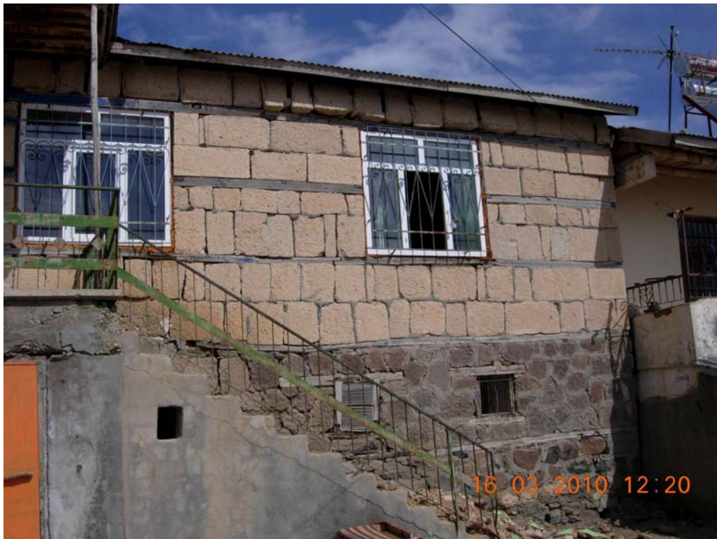
Figure 31: Two storey house, with a combination of heavy stones in the ground floor, and light stones in the upper floor, Okcular village
