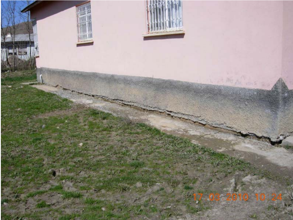
Figure 71: RC house, built by government, after 2003 Bingol earthquake, Incedal village
