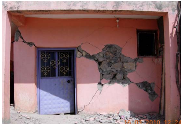
Figure 82: Wide cracks following the mortar, Okcular village
