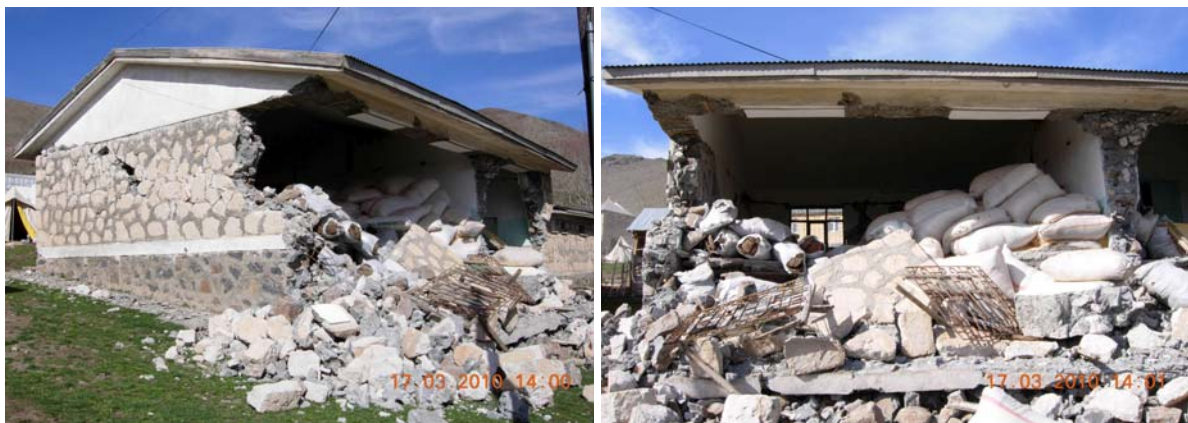
Figure 73: Out of plane failure in one story, stone school building (being used for storage), Gocmezler village
