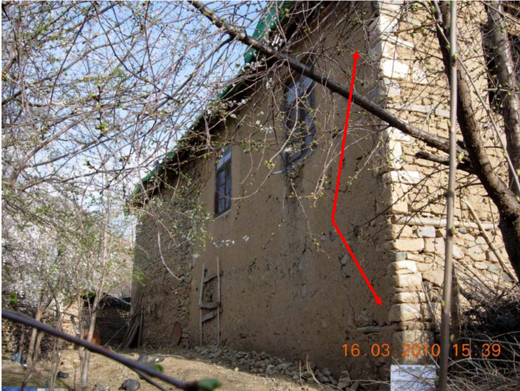
Figure 25: Two storey soil brick house with a stall in the ground floor (only lintel application ever seen in that area), side view, Beyhani
