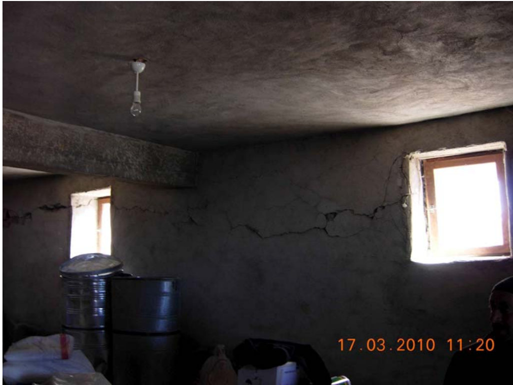
Figure 43: Inside view of two storeys mixed structural system, RC beam, RC slab, heavy stone wall, Okcular village
